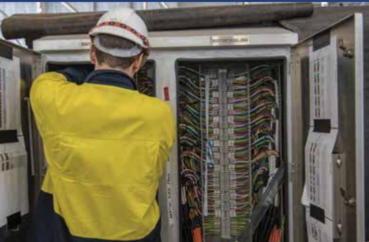
ELECTRICAL, INSTRUMENTATION & CONTROL
