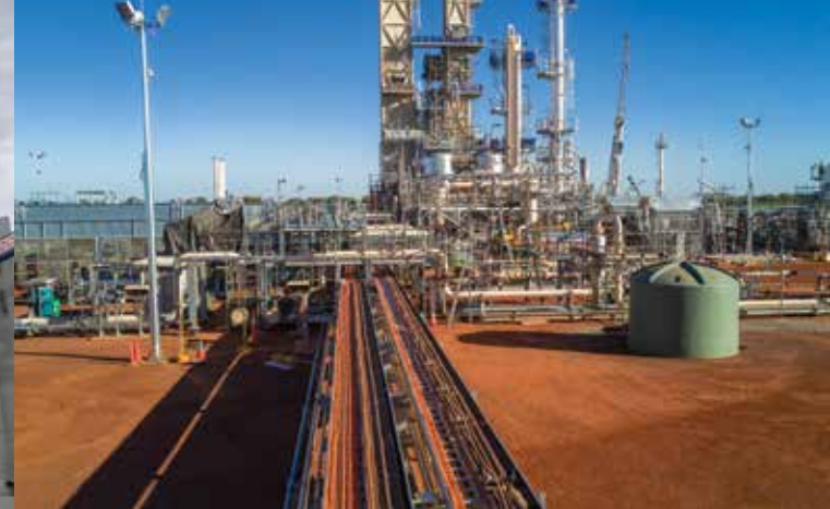
STRUCTURAL, MECHANICAL & PIPING
